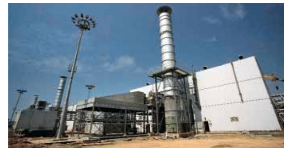
Gas reinjection compressors at Unit 2, August 2002.
